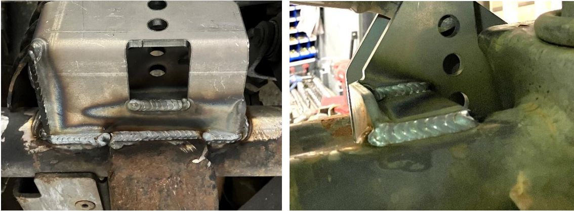
Figures 17 and 18. Completed Welds on the Top and Bottom of the Track Bar Bracket
