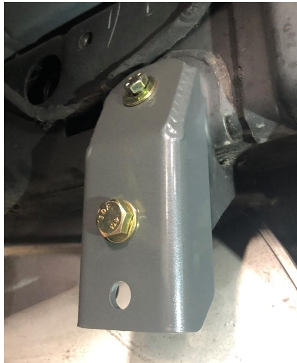
Figure 3. Loosely Installed 8708 Bracket.
